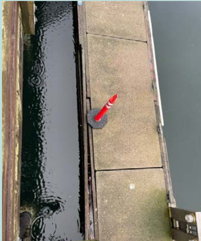
Winter storm caused damage to finger piers; siding is separating from float.
