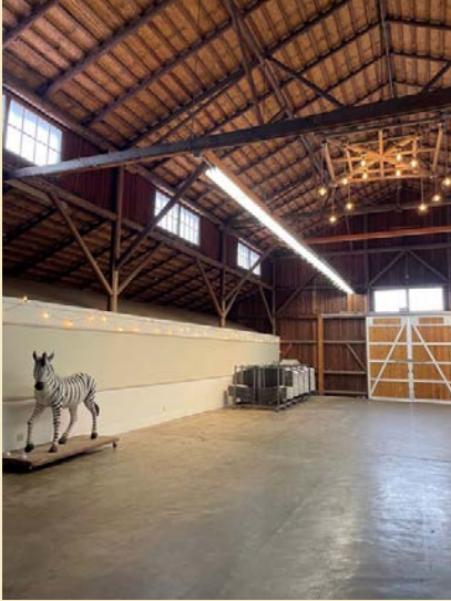
The Pole building is a great event space, but needs additional electrical power and heat.
