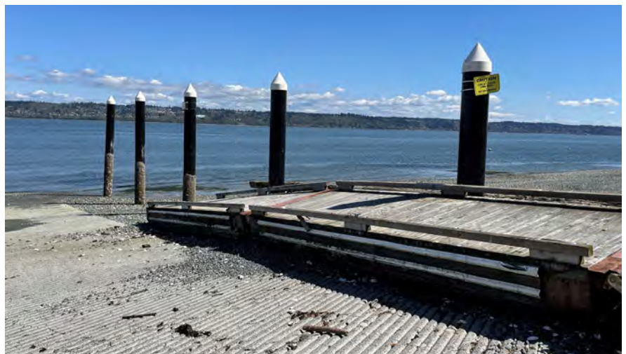
Floating docks along the boat launch are prepared for installation in April after being removed for the winter.
