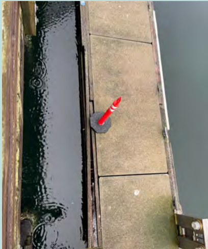
Winter storm caused damage to finger piers; siding is separating from float.
