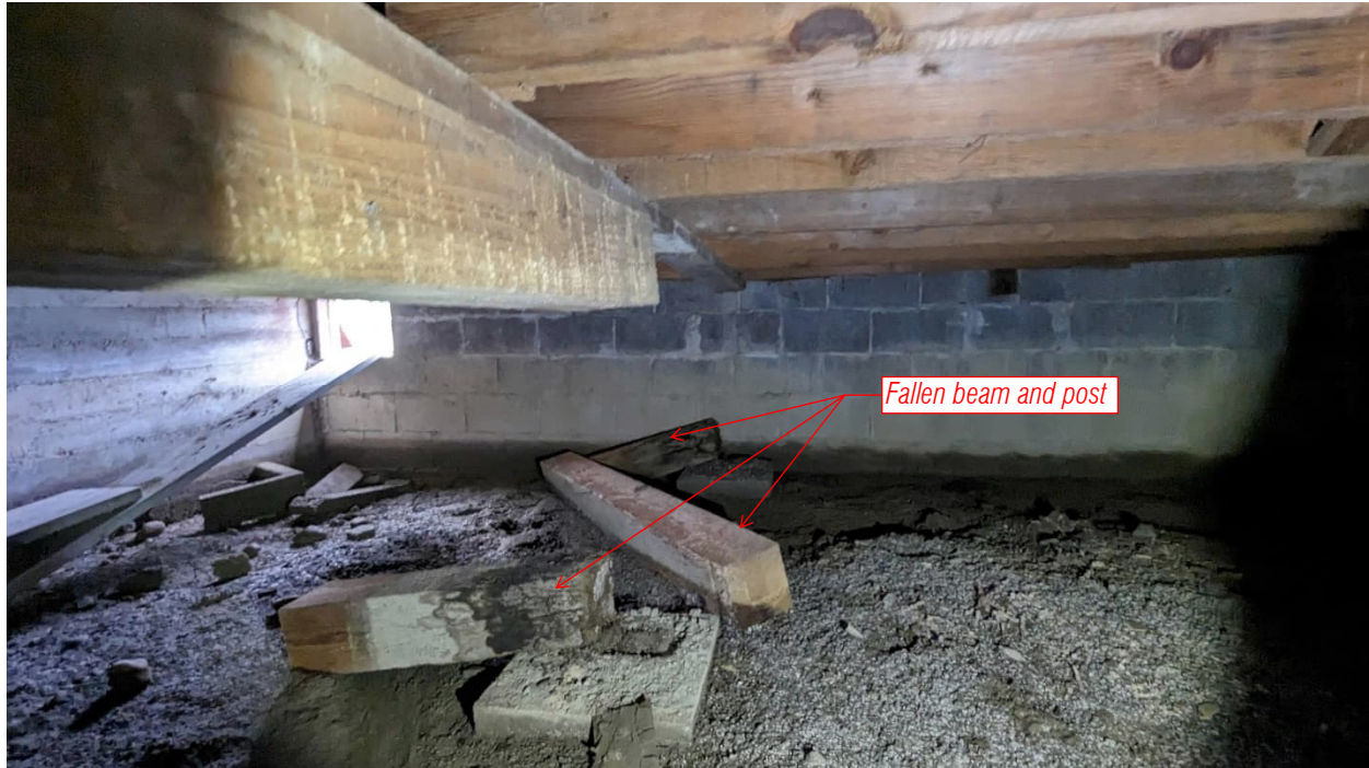
Figure 1 – Fallen Post and Beams
