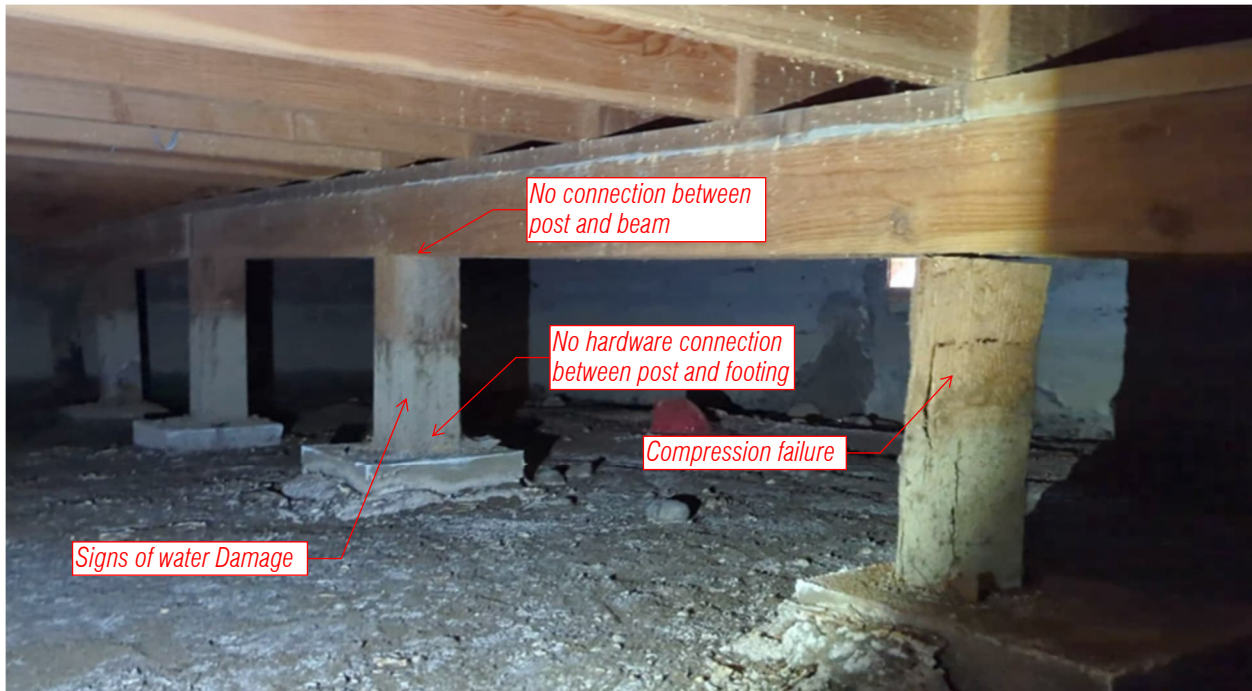
Figure 2 – Water Damage and Post Failure
